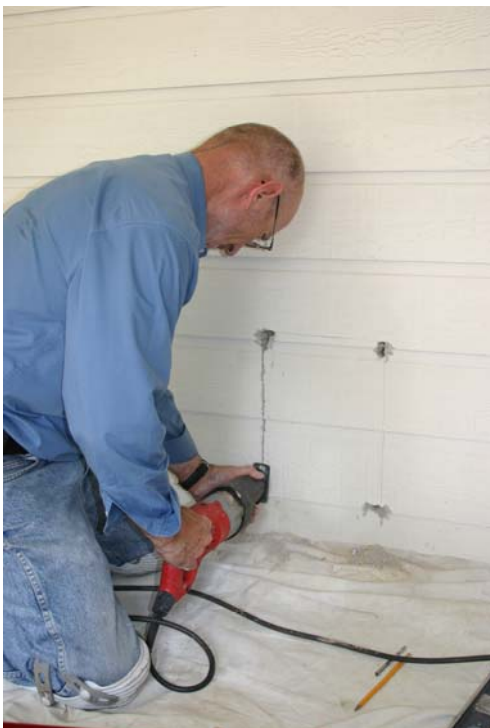
A reciprocating saw easily cuts the exterior hole, although other types of saw can be used.
