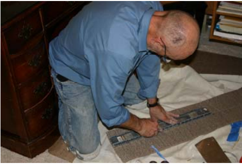
Measure and cut the carpet to the correct width for the tunnel
